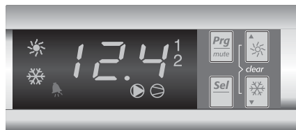
Figure - Digital controller
